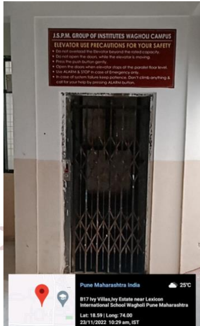
Fig. 15 Lift in building A of ICOER
