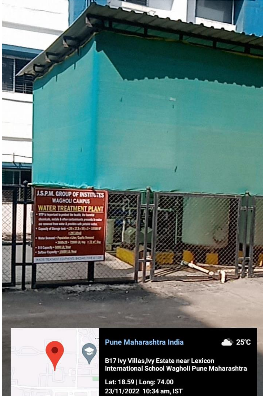
Fig. 9 Water Treatment Plant at at ICOER
