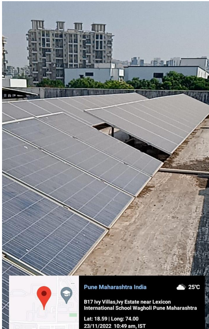
Fig. 1 Solar panle on roof of building-C
